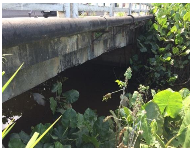
Fig. 6: Inadequate mounting of pipes on deck, increasing the damages on the concrete
