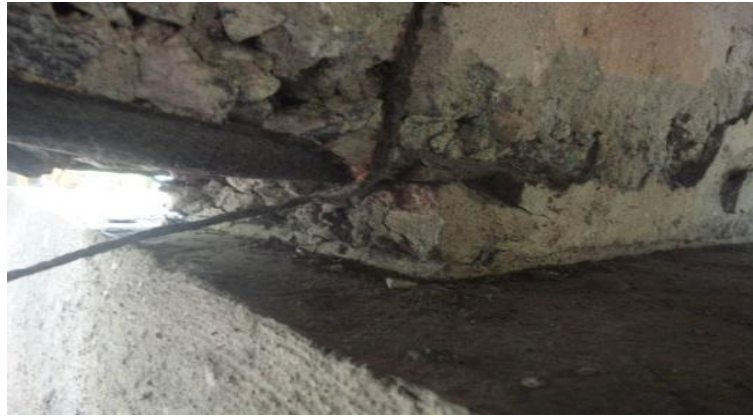
Fig. 9: Crushing of the concrete and bearings of one of the beams
