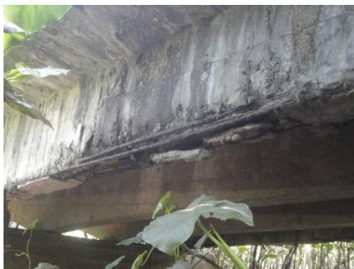
Fig. 4: Loss of concrete sections and bending rebar in external girders
