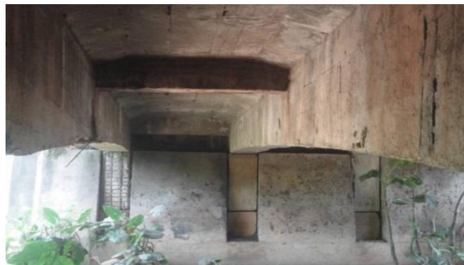
Fig. 8: Collapse of one of the pendulums type bearings one of the girders.
