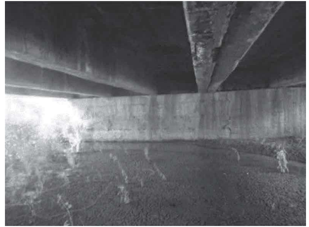
Figure 11. Widening without consolidating the old structure.
