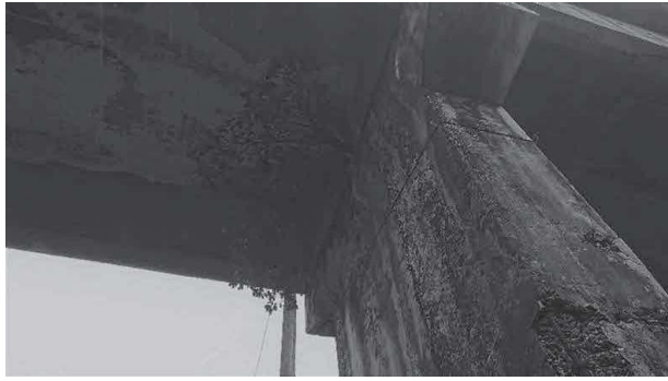
Figure 8. Presence of sparse vegetation, general seepage, efflorescence and corrosion of reinforcement on one side of the walkway's pillar.
