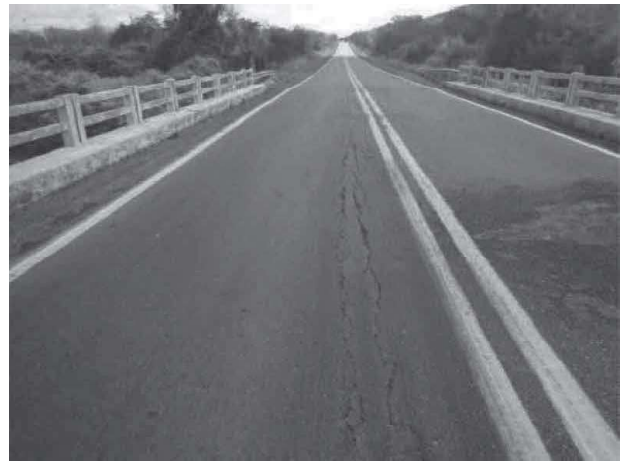
Figure 12. Subsidence in a traffic lane on the bridge.
