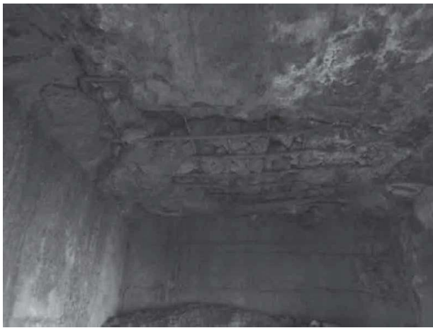
Figure 9. Severe deterioration of the bottom part of the deck due to the presence of holes in the concrete and efflorescence.
