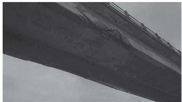
Figure 6. Stringers in the central walkway containing reinforcement bars and shearing partly destroyed by vehicle impact.
