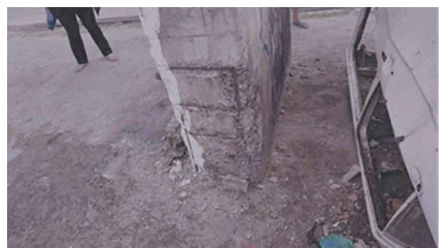
Figure 7. Corrosion of reinforcements at the bottom of one lateral pillar surface of the structure.
