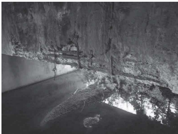
Figure 10. Severely corroded reinforcement bars in one of the bridge stringers.
